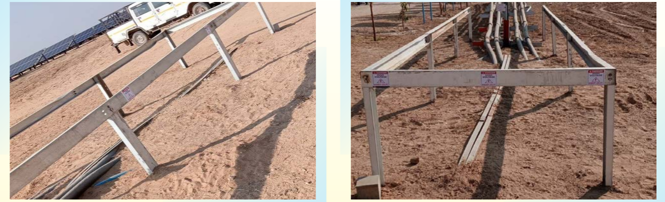
Damaged Purlin used for 33 KV Cable Tray Barricading.
